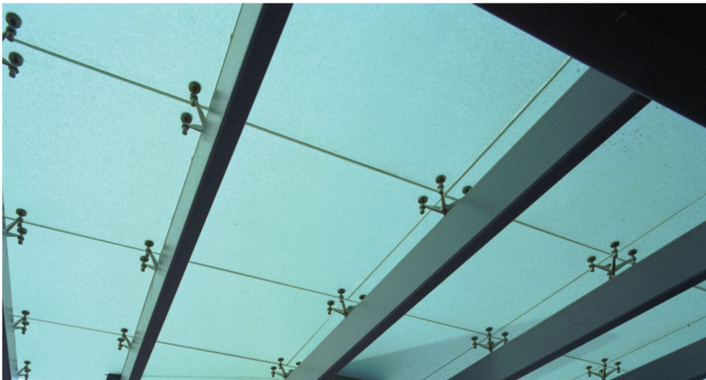
University of Michigan Skylight System
