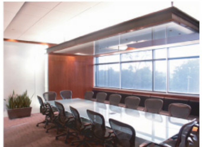
Colliers International - Custom laminated/blast lighting diffusion assembly, Southfield, MI
